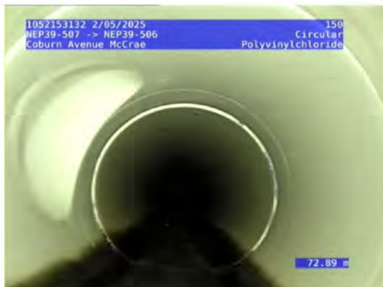
7, 00:16:36, 72.89 Junction, unlined, open, Height/Diameter (mm): 100 at 10 o'clock
