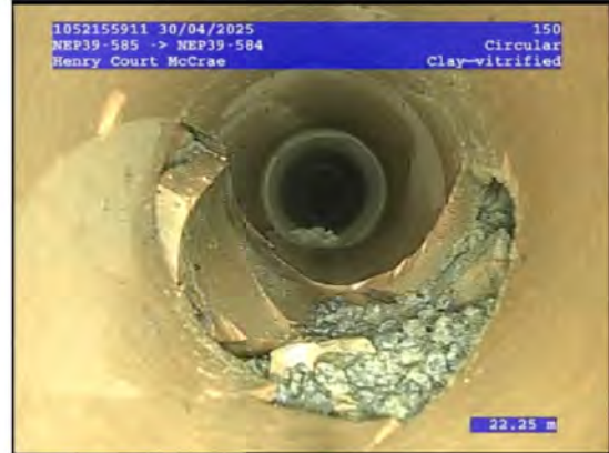
6, 00:10:21, 22.24 Conduit broken as a result of an exceptional event, e.g. external trauma, length of break: 500mm from 2 o'clock to 11 o'clock
