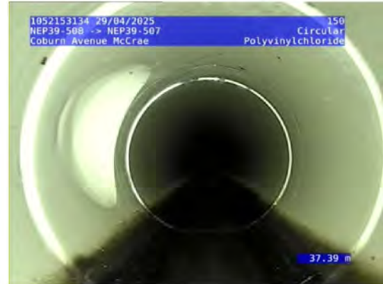
10, 00:10:26, 37.39 Junction, unlined, open, Height/Diameter (mm): 100 at 10 o'clock
