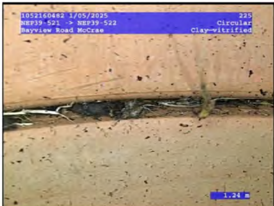
3, 00:01:21, 1.24 Recently cut fine roots-a relatively small number of cut minor roots remain, Obstruction: 10%, at joint from 12 o'clock to 12 o'clock
