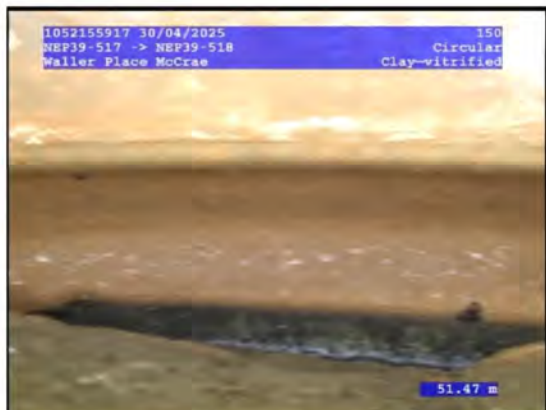
15, 00:20:09, 51.47 Seal is visibly displaced and/or damaged but not intruding into the conduit from 9 o'clock to 11 o'clock
