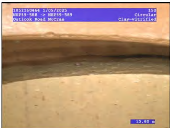
3, 00:13:34, 13.80 Joint displaced angular at 3 o'clock
