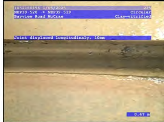
2, 00:00:58, 0.47 Joint displaced longitudinally, 10mm
