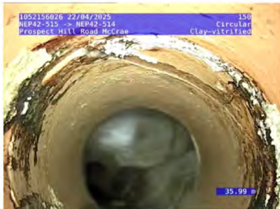
3, 00:10:52, 35.99 Breaking, all pieces are present but some of them are visibly displaced from position, length of break: 100mm from 10 o'clock to 2 o'clock
