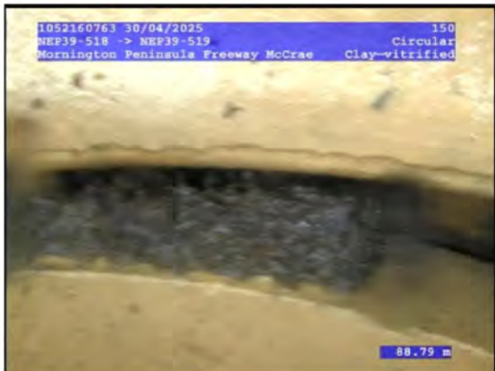
7, 00:44:03, 88.79 Joint displaced angular at 3 o'clock
