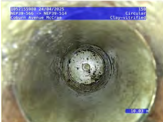
5, 00:05:19, 10.03 Junction, unlined, open, Height/Diameter (mm): 100 at 12 o'clock
