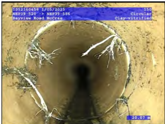
7, 00:06:58, 20.07 Recently cut interwoven mass of mostly fine roots leaving a beard of roots, at joint from 12 o'clock to 12 o'clock
