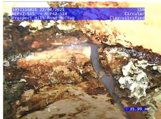
4, 00:11:00, 35.99 Infiltration, gushing, at joint from 11 o'clock to 1 o'clock
