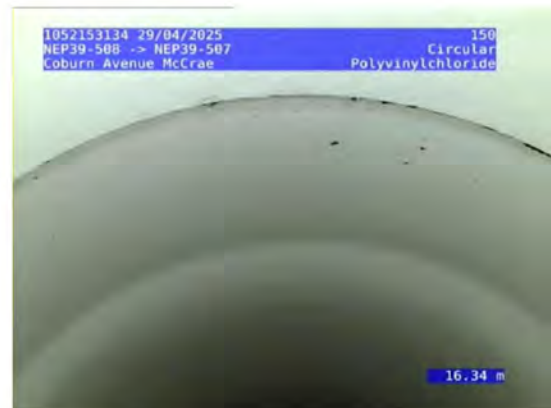
4, 00:05:02, 16.34 Joint displaced longitudinally, 40mm
