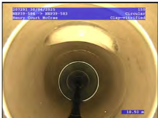
3, 00:05:23, 10.50 Junction, unlined, open, Height/Diameter (mm): 100 at 12 o'clock
