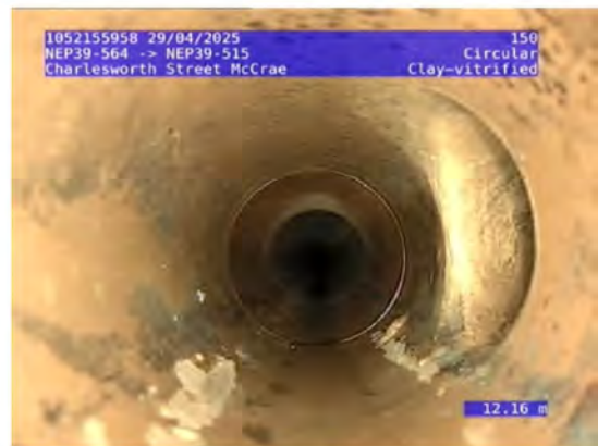
4, 00:04:57, 12.16 Junction, unlined, open, Height/Diameter (mm): 100 at 2 o'clock
