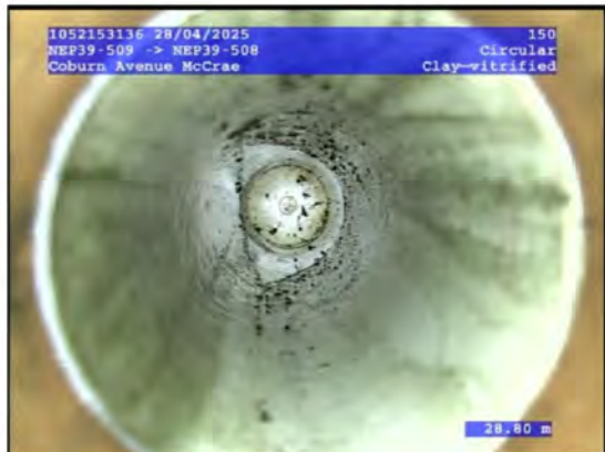
3, 00:09:45, 28.80 Junction, unlined, open, Height/Diameter (mm): 100 at 12 o'clock
