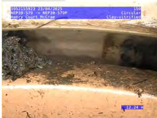
5, 00:06:23, 12.24 Joint displaced longitudinally, 20mm
