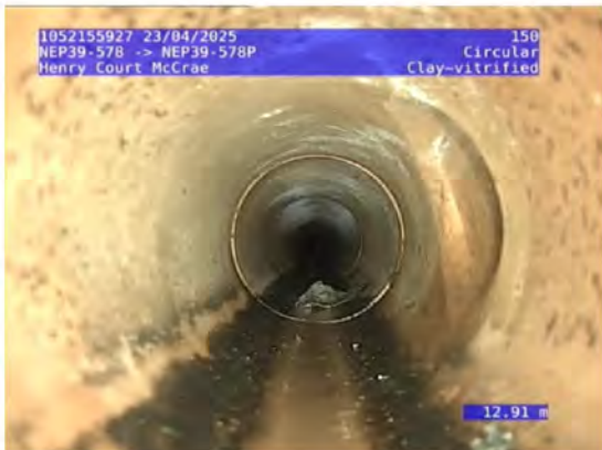
3, 00:04:59, 12.91 Junction, unlined, open, Height/Diameter (mm): 100 at 2 o'clock
