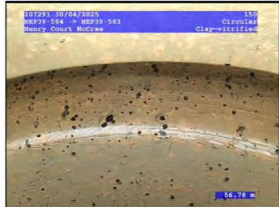
10, 00:25:50, 56.78 Joint displaced longitudinally, 20mm
