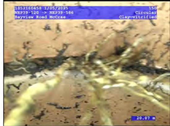
6, 00:06:58, 20.07 Recently cut interwoven mass of mostly fine roots leaving a beard of roots, at joint from 12 o'clock to 12 o'clock
