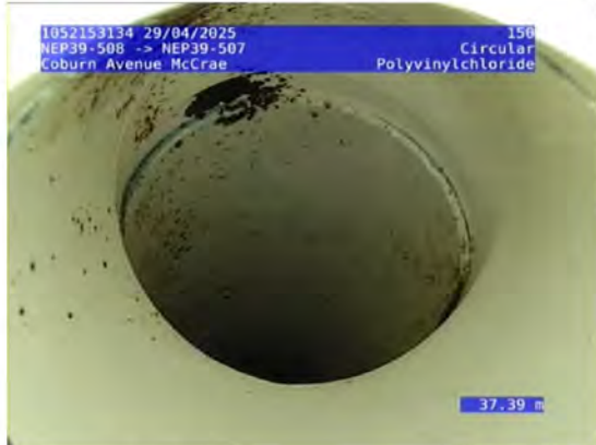
9, 00:10:26, 37.39 Junction, unlined, open, Height/Diameter (mm): 100 at 10 o'clock
