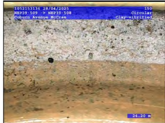
2, 00:08:03, 24.20 Joint displaced longitudinally, 40mm
