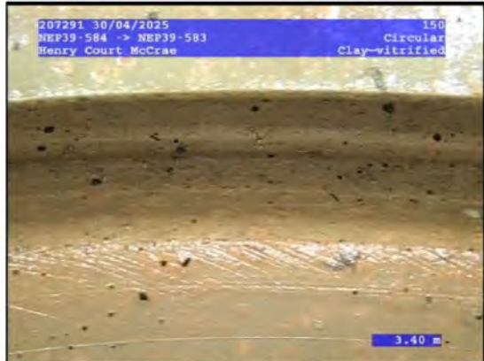
1, 00:02:15, 3.41 Joint displaced longitudinally, 10mm
