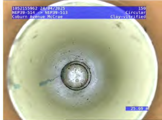
2, 00:08:07, 25.69 Junction, unlined, open, Height/Diameter (mm): 100 at 12 o'clock
