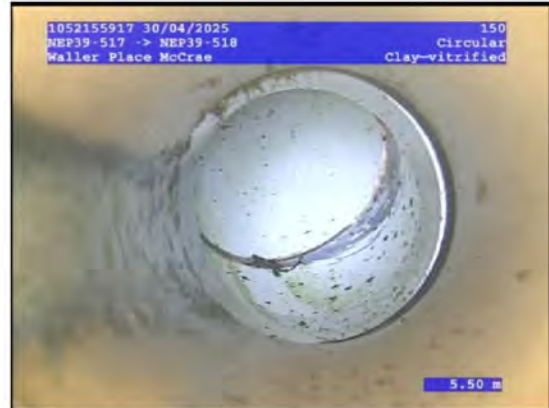
10, 00:04:32, 5.50 Connection, unlined, connection appears to be open, Height/Diameter (mm): 100 at 10 o'clock
