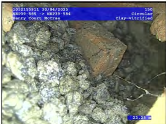
7, 00:10:42, 22.25 Void visible through defect, at joint
