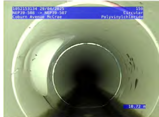
6, 00:05:33, 18.72 Junction, unlined, open, Height/Diameter (mm): 100 at 10 o'clock
