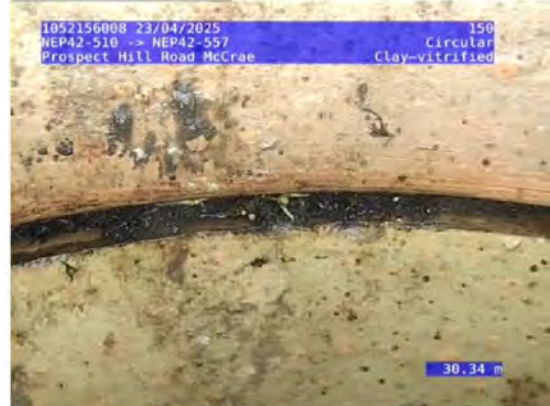
2, 00:09:04, 30.34 Recently cut interwoven mass of mostly fine roots leaving a beard of roots, at joint from 3 o'clock to 9 o'clock
