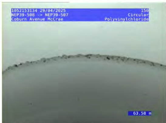
15, 00:16:48, 63.58 Joint displaced longitudinally, 30mm
