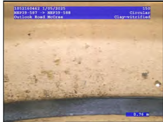
2, 00:00:56, 0.76 Joint displaced longitudinally, 60mm
