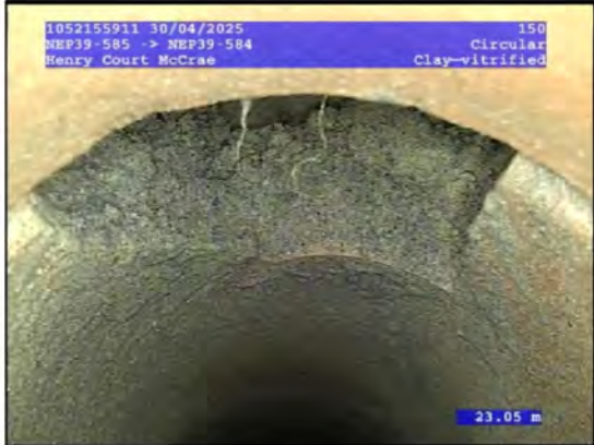
13, 00:12:37, 23.05 Void visible through defect, at joint
