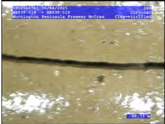
9, 00:45:52, 89.73 Circumferential cracking, width: 1.5mm from 12 o'clock to 12 o'clock
