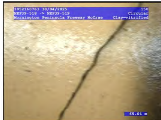
4, 00:24:20, 65.04 Simple cracking, width: 1mm from 4 o'clock to 8 o'clock
