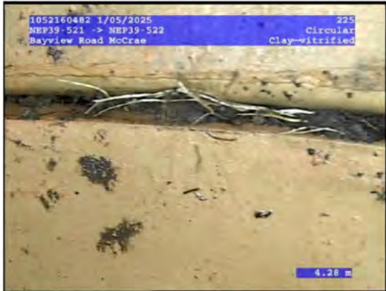
5, 00:02:55, 4.28 Recently cut fine roots-a relatively small number of cut minor roots remain, at joint from 3 o'clock to 9 o'clock
