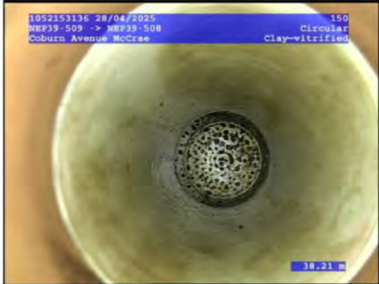
5, 00:13:48, 38.21 Junction, unlined, open, Height/Diameter (mm): 100 at 12 o'clock
