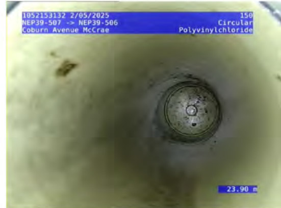
2, 00:05:29, 23.90 Junction, unlined, open, Height/Diameter (mm): 100 at 12 o'clock
