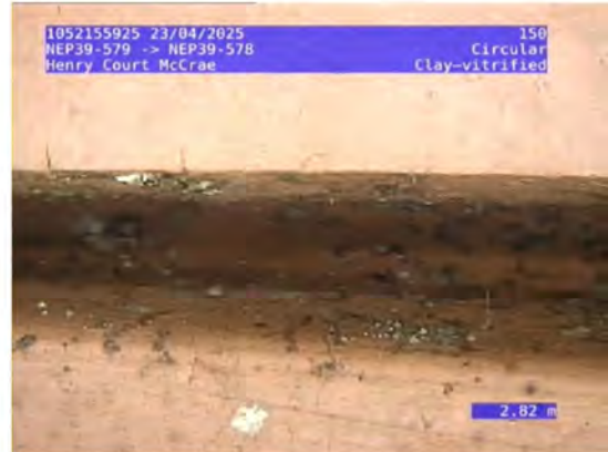
2, 00:01:53, 2.82 Joint displaced angular at 3 o'clock
