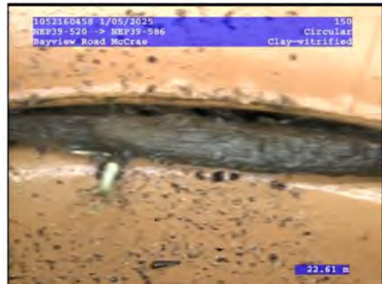
8, 00:07:55, 22.61 Recently cut tap roots, a small number of cut major roots (10mm or greater) is evident, at joint from 2 o'clock to 3 o'clock
