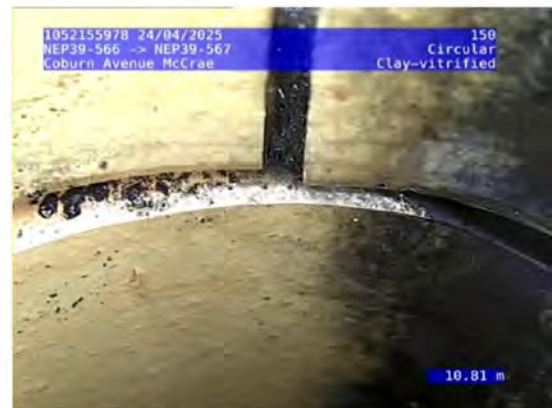
4, 00:04:09, 10.81 Breaking, all pieces are present but some of them are visibly displaced from position, length of break: 200mm from 4 o'clock to 11 o'clock
