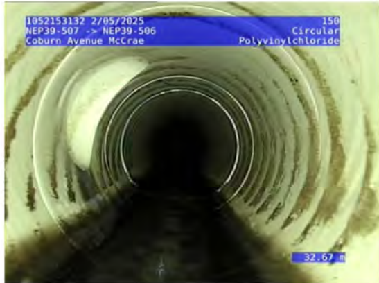
5, 00:08:17, 32.67 Junction, unlined, open, Height/Diameter (mm): 100 at 10 o'clock
