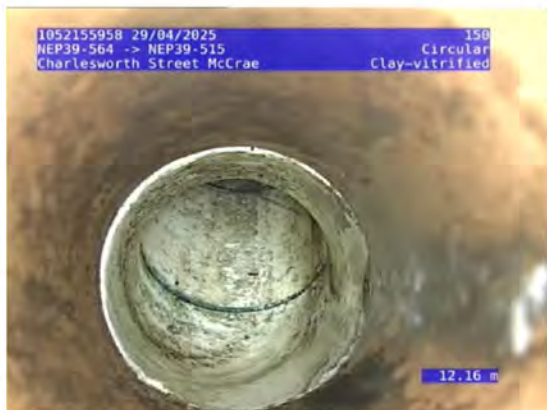
3, 00:04:57, 12.16 Junction, unlined, open, Height/Diameter (mm): 100 at 2 o'clock
