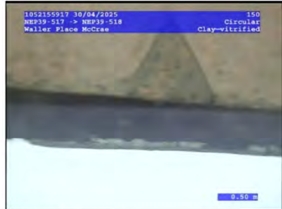
2, 00:01:13, 0.50 Change of conduit material. New material, Polyvinyl chloride, at joint
