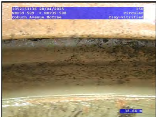
7, 00:14:35, 38.64 Joint displaced longitudinally, 10mm
