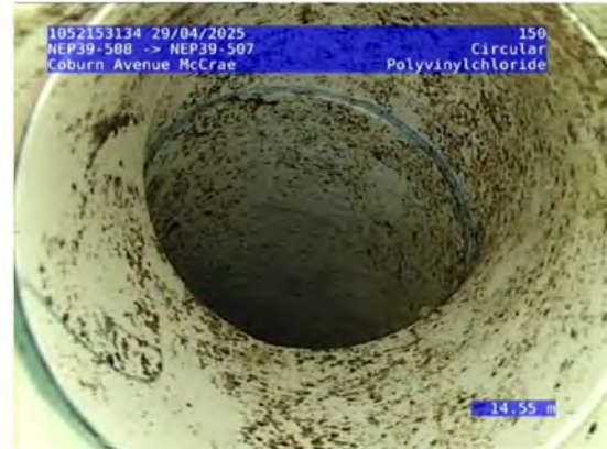
2, 00:03:50, 14.55 Junction, unlined, open, Height/Diameter (mm): 100 at 10 o'clock
