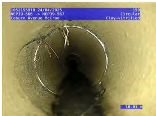
3, 00:03:37, 10.80 Recently cut interwoven mass of mostly fine roots leaving a beard of roots, at joint from 12 o'clock to 12 o'clock
