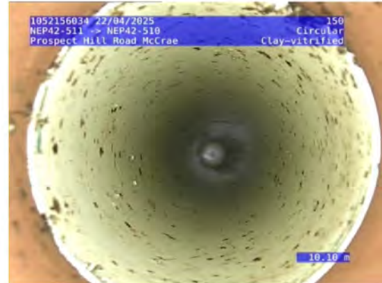
2, 00:03:51, 10.10 Junction, unlined, open, Height/Diameter (mm): 100 at 12 o'clock
