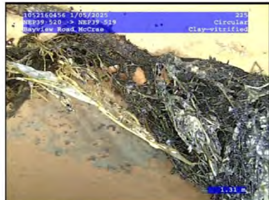
4, 00:02:11, 1.31 Recently cut interwoven mass of mostly fine roots leaving a beard of roots, Obstruction: 70%, at joint from 12 o'clock to 12 o'clock
