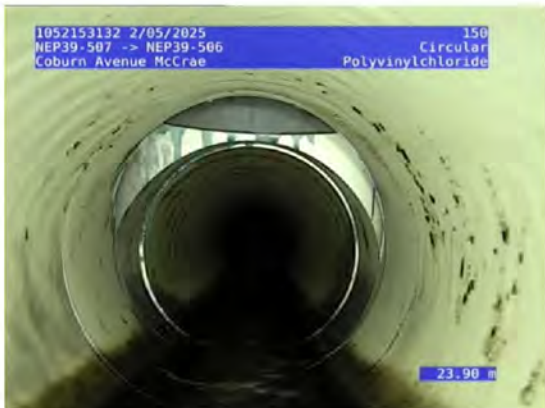
3, 00:05:29, 23.90 Junction, unlined, open, Height/Diameter (mm): 100 at 12 o'clock
