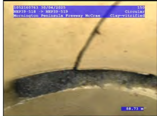
6, 00:43:40, 88.73 Simple cracking, at joint, width: 1mm from 9 o'clock to 10 o'clock
