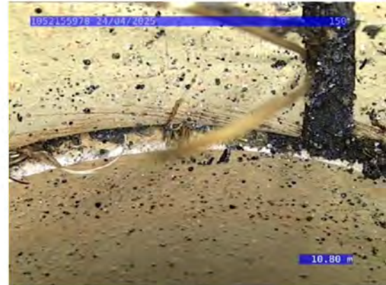
2, 00:03:37, 10.80 Recently cut interwoven mass of mostly fine roots leaving a beard of roots, at joint from 12 o'clock to 12 o'clock
