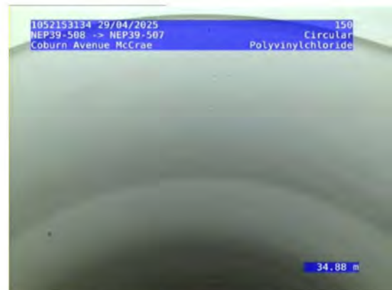
8, 00:09:50, 34.88 Joint displaced longitudinally, 50mm
