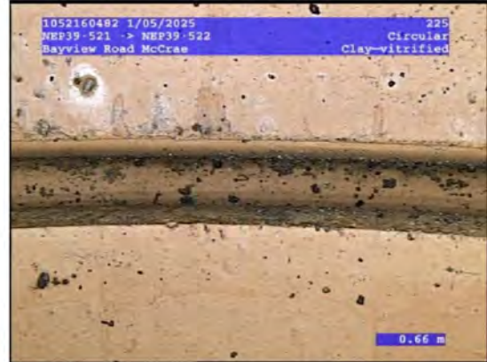
2, 00:00:59, 0.66 Joint displaced longitudinally, 10mm
