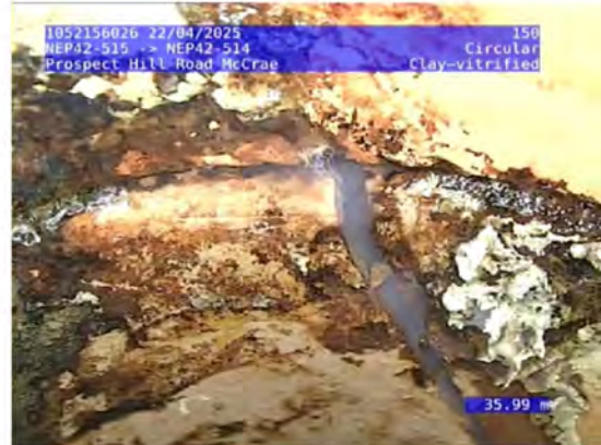
2, 00:10:52, 35.99 Breaking, all pieces are present but some of them are visibly displaced from position, length of break: 100mm from 10 o'clock to 2 o'clock
