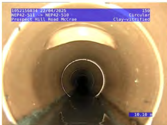
3, 00:03:51, 10.10 Junction, unlined, open, Height/Diameter (mm): 100 at 12 o'clock
