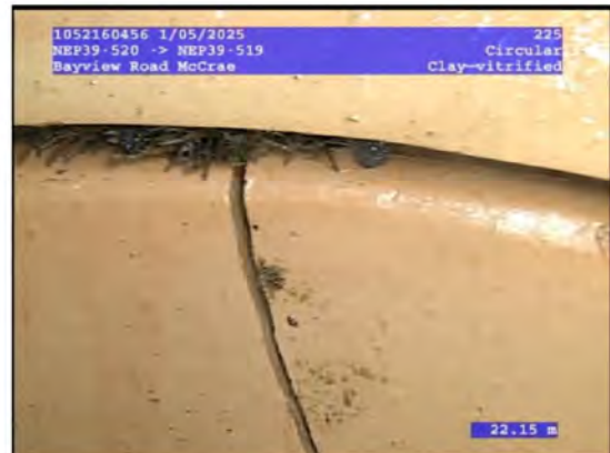
4, 00:07:01, 22.15 Simple cracking, at joint, width: 1mm from 3 o'clock to 8 o'clock
