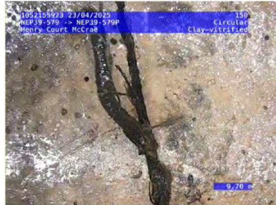
2, 00:05:05, 9.70 Longitudinal cracking, at joint, width: 2mm at 8 o'clock
