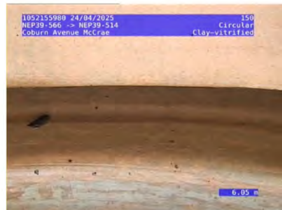
4, 00:03:34, 6.05 Joint displaced longitudinally, 10mm
