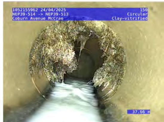
4, 00:12:06, 37.66 Recently cut interwoven mass of mostly fine roots leaving a beard of roots, Obstruction: 20%, at joint from 12 o'clock to 12 o'clock
