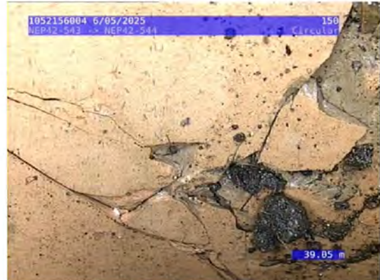
6, 00:17:19, 39.05 Cracking multiple or complex (s), at joint, width: 1mm from 4 o'clock to 7 o'clock
