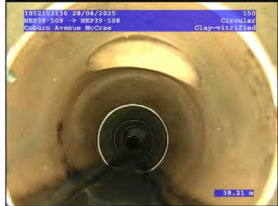
6, 00:13:48, 38.21 Junction, unlined, open, Height/Diameter (mm): 100 at 12 o'clock
