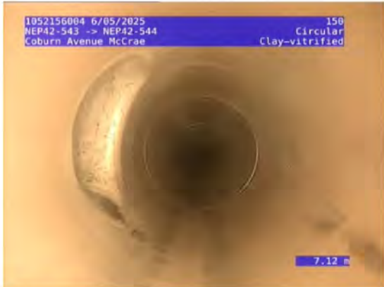
5, 00:05:40, 7.12 Junction, unlined, open, Height/Diameter (mm): 100 at 10 o'clock
