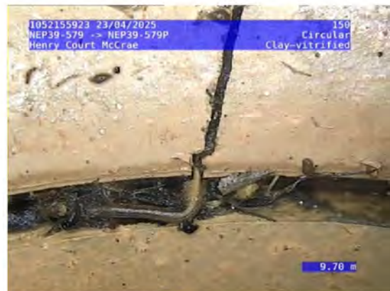
4, 00:05:32, 9.70 Recently cut interwoven mass of mostly fine roots leaving a beard of roots, Obstruction: 10%, at joint from 3 o'clock to 9 o'clock
