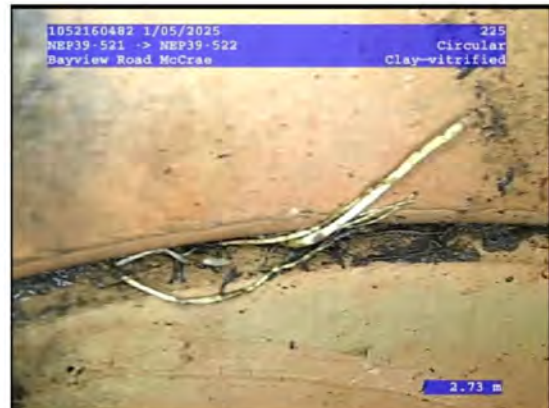
4, 00:02:02, 2.73 Recently cut fine roots-a relatively small number of cut minor roots remain, Obstruction: 10%, at joint from 3 o'clock to 9 o'clock
