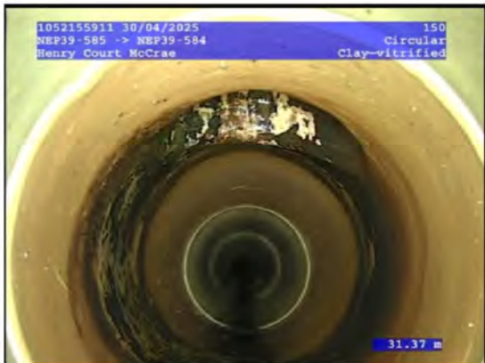
15, 00:15:38, 31.37 Junction, unlined, open, Height/Diameter (mm): 100 at 12 o'clock
