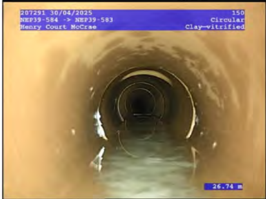
5, 00:11:39, 26.74 Ponding of water with or without flow turbid or discoloured water, 10-20 mm
