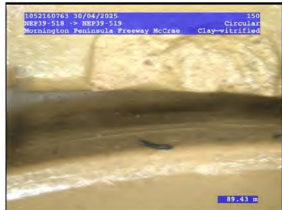
8, 00:45:20, 89.43 Joint displaced angular at 3 o'clock
