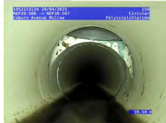
14, 00:15:36, 59.54 Junction, unlined, open, Height/Diameter (mm): 100 at 12 o'clock / 150 junction into 100 connection
