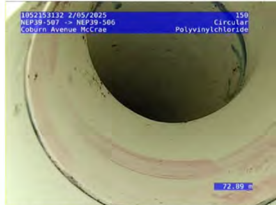
6, 00:16:36, 72.89 Junction, unlined, open, Height/Diameter (mm): 100 at 10 o'clock
