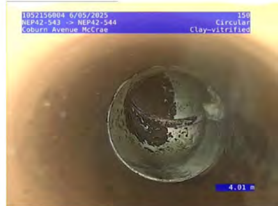
2, 00:04:03, 4.01 Junction, unlined, open, Height/Diameter (mm): 100 at 2 o'clock
