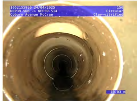
6, 00:05:19, 10.03 Junction, unlined, open, Height/Diameter (mm): 100 at 12 o'clock
