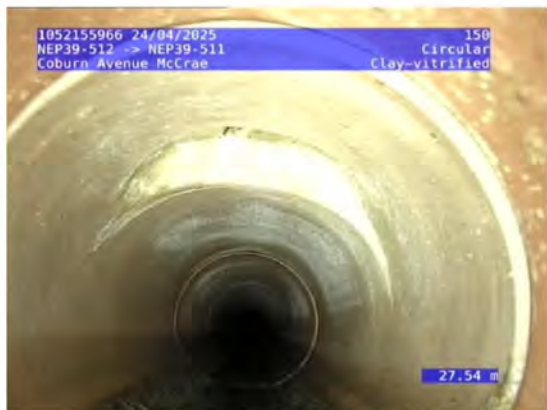
3, 00:09:04, 27.54 Junction, unlined, open, Height/Diameter (mm): 100 at 12 o'clock
