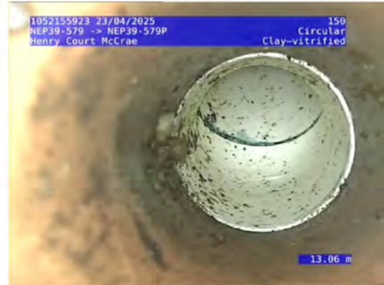
6, 00:06:53, 13.06 Junction, unlined, open, Height/Diameter (mm): 100 at 9 o'clock
