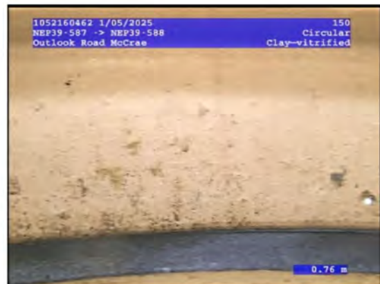
4, 00:01:04, 0.76 Seal is visibly displaced and/or damaged but not intruding into the conduit from 12 o'clock to 12 o'clock
