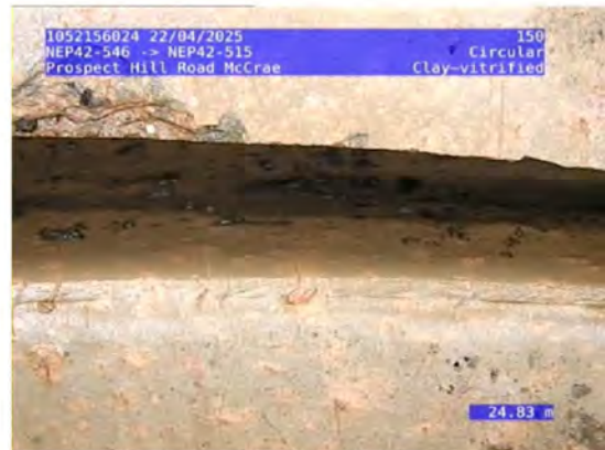
4, 00:08:25, 24.83 Joint displaced angular at 3 o'clock
