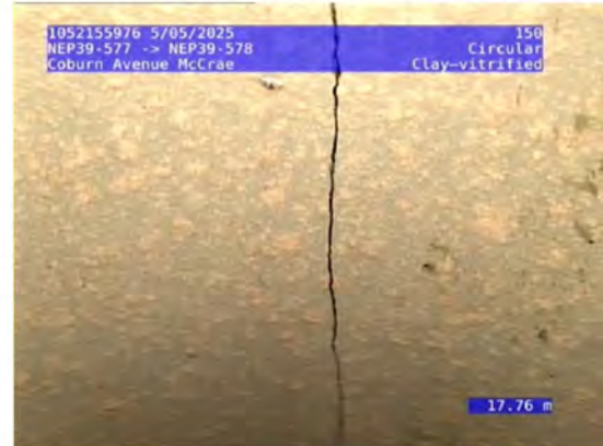
2, 00:06:13, 17.76 Longitudinal cracking, at joint, width: 0.5mm at 2 o'clock
