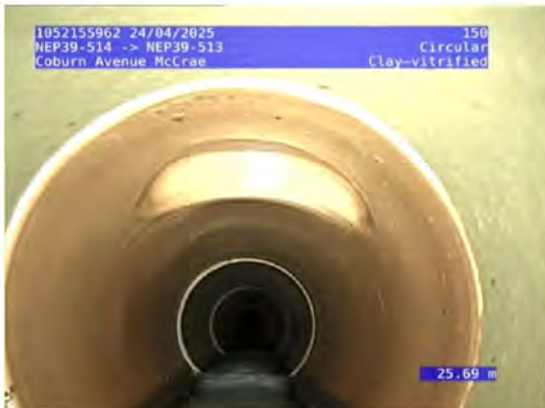
3, 00:08:07, 25.69 Junction, unlined, open, Height/Diameter (mm): 100 at 12 o'clock
