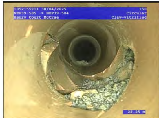
8, 00:10:42, 22.25 Void visible through defect, at joint
