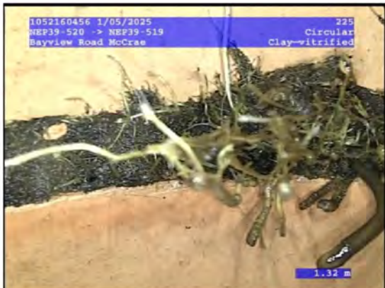
3, 00:01:23, 1.32 Recently cut interwoven mass of mostly fine roots leaving a beard of roots, Obstruction: 10%, at joint from 12 o'clock to 12 o'clock
