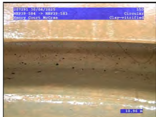
4, 00:06:09, 10.96 Joint displaced longitudinally, 10mm
