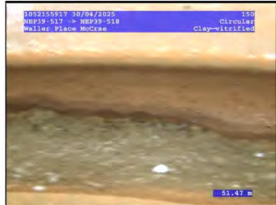
14, 00:19:55, 51.47 Surface damage, spalling of a masonry or VC conduit including localised chipping, at joint, Obstruction: 20% from 12 o'clock to 12 o'clock
