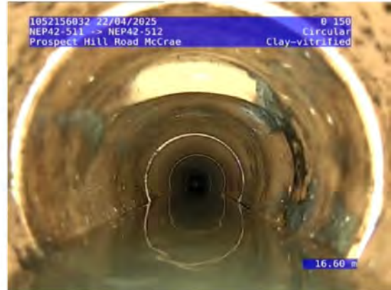
6, 00:06:25, 16.60 Junction, unlined, open, Height/Diameter (mm): 100 at 12 o'clock
