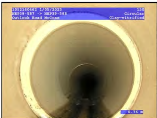
3, 00:00:56, 0.76 Joint displaced longitudinally, 60mm
