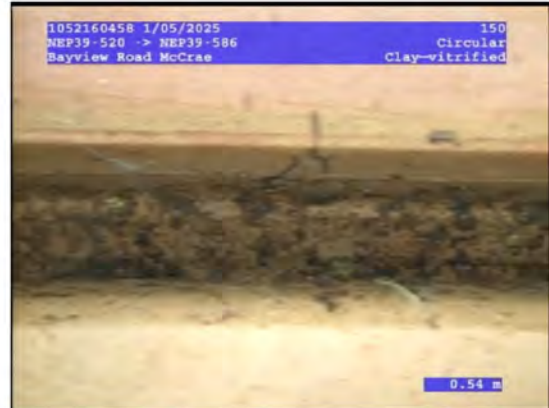
2, 00:00:59, 0.54 Joint displaced longitudinally, 10mm
