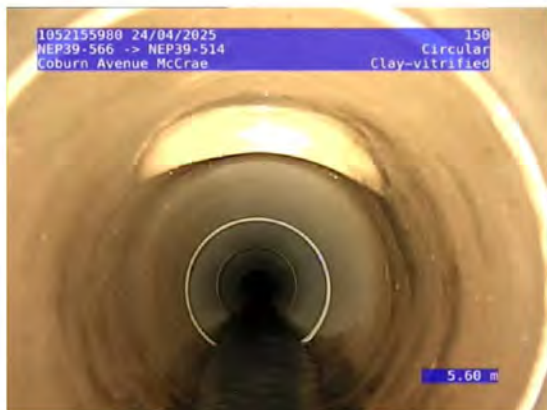
3, 00:02:48, 5.60 Junction, unlined, open, Height/Diameter (mm): 100 at 12 o'clock
