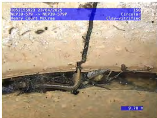
3, 00:05:22, 9.70 Longitudinal cracking, at joint, width: 2mm at 4 o'clock
