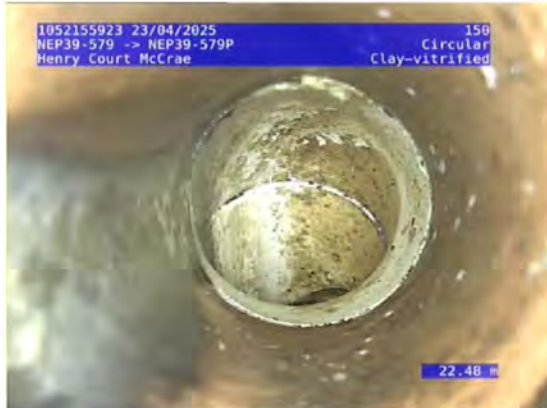
9, 00:10:32, 22.48 Junction, unlined, open, Height/Diameter (mm): 100 at 10 o'clock
