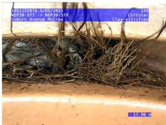
3, 00:06:48, 17.90 Recently cut interwoven mass of mostly fine roots leaving a beard of roots, at joint from 2 o'clock to 3 o'clock
