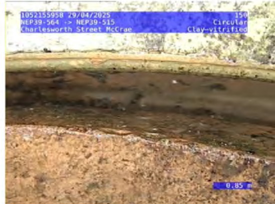
2, 00:01:13, 0.85 Joint displaced angular at 3 o'clock
