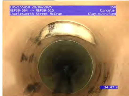
6, 00:12:16, 34.47 Junction, unlined, open, Height/Diameter (mm): 100 at 12 o'clock
