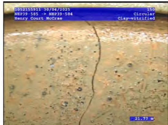
4, 00:09:43, 21.77 Longitudinal cracking, at joint, width: 1mm at 8 o'clock
