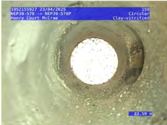
5, 00:08:21, 23.59 Junction, unlined, open, Height/Diameter (mm): 100 at 2 o'clock
