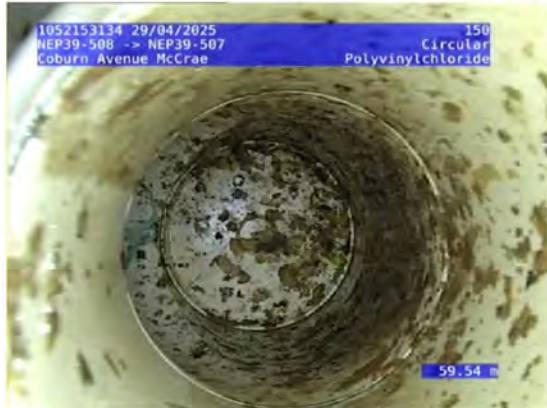
13, 00:15:36, 59.54 Junction, unlined, open, Height/Diameter (mm): 100 at 12 o'clock / 150 junction into 100 connection
