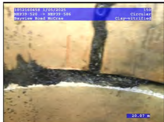
4, 00:06:46, 20.07 Cracking multiple or complex (s), at joint, width: 3mm from 12 o'clock to 12 o'clock
