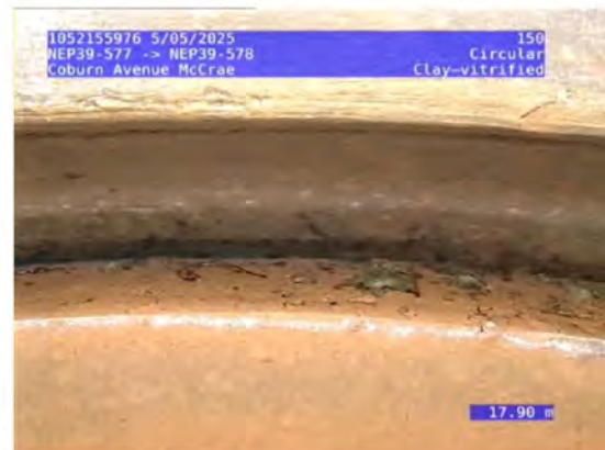
4, 00:07:00, 17.90 Joint displaced longitudinally, 10mm
