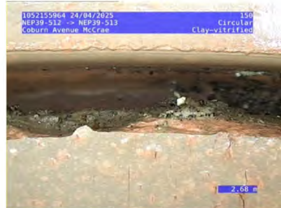
2, 00:01:42, 2.68 Joint displaced longitudinally, 10mm
