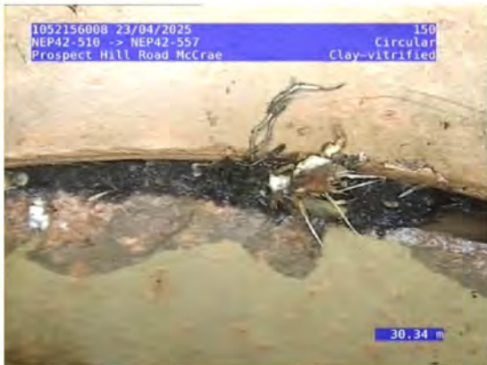
3, 00:09:04, 30.34 Recently cut interwoven mass of mostly fine roots leaving a beard of roots, at joint from 3 o'clock to 9 o'clock
