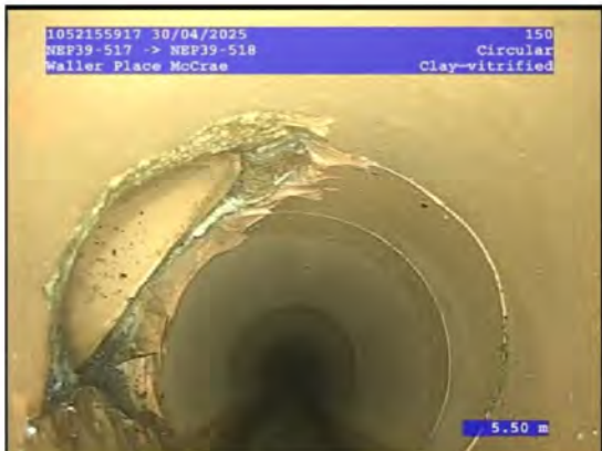
11, 00:04:32, 5.50 Connection, unlined, connection appears to be open, Height/Diameter (mm): 100 at 10 o'clock
