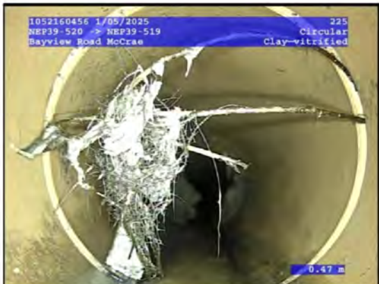
3, 00:01:26, 0.47 Recently cut interwoven mass of mostly fine roots leaving a beard of roots, Obstruction: 30%, at joint from 12 o'clock to 12 o'clock
