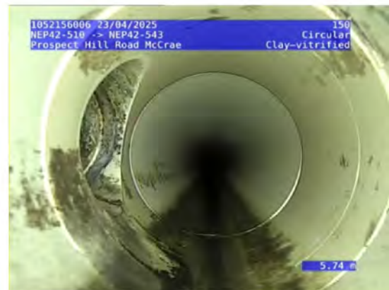
4, 00:02:14, 5.74 Junction, unlined, open, Height/Diameter (mm): 100 at 9 o'clock
