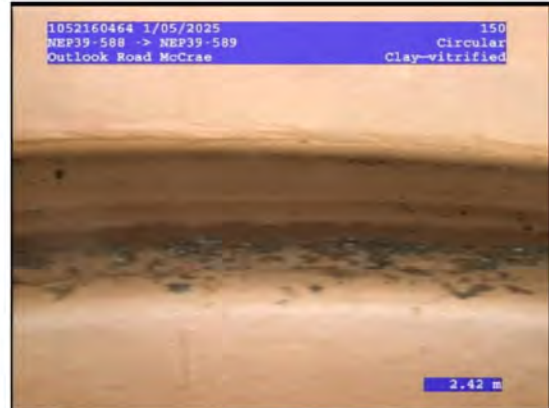
2, 00:04:09, 2.42 Joint displaced longitudinally, 10mm
