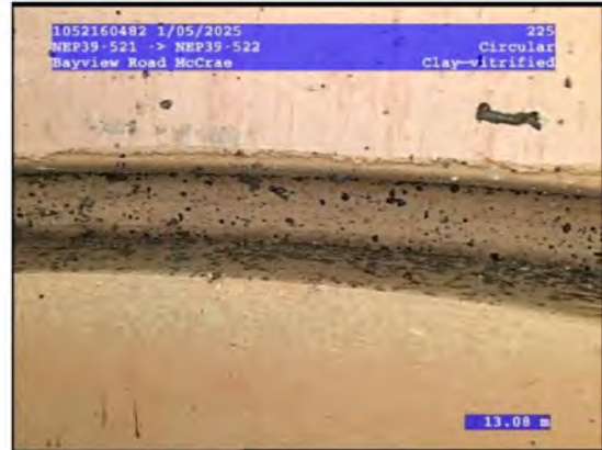
6, 00:05:51, 13.08 Joint displaced longitudinally, 10mm
