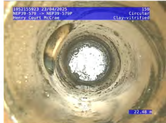
10, 00:10:32, 22.48 Junction, unlined, open, Height/Diameter (mm): 100 at 10 o'clock
