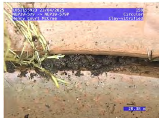
8, 00:09:19, 20.38 Recently cut interwoven mass of mostly fine roots leaving a beard of roots, at joint from 12 o'clock to 12 o'clock
