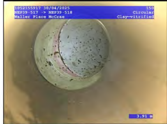
6, 00:03:03, 3.91 Connection, unlined, connection appears to be open, Height/Diameter (mm): 100 at 2 o'clock
