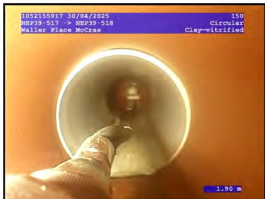
3, 00:01:13, 0.50 Change of conduit material. New material, Polyvinyl chloride, at joint
