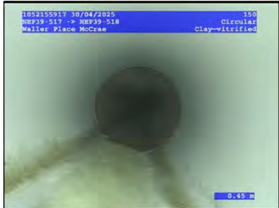
1, 00:00:25, 0.45 Water flow at constant depth, turbid or discoloured water, <5% / Pulsating
