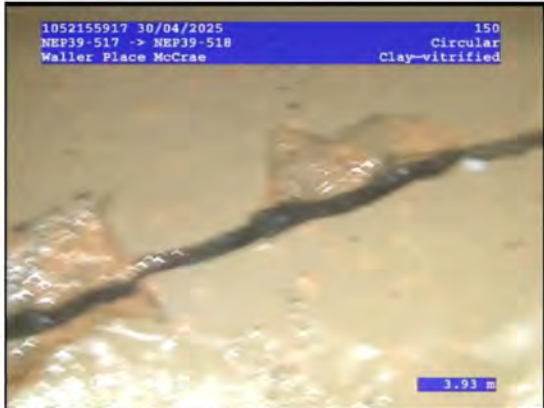
9, 00:03:18, 3.91 Cracking multiple or complex (s), at joint, width: 1.5mm from 4 o'clock to 10 o'clock / from connection
