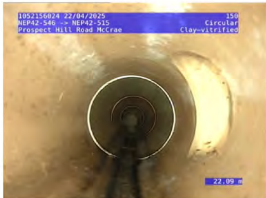
3, 00:07:05, 22.09 Junction, unlined, open, Height/Diameter (mm): 100 at 2 o'clock
