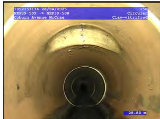
4, 00:09:45, 28.80 Junction, unlined, open, Height/Diameter (mm): 100 at 12 o'clock
