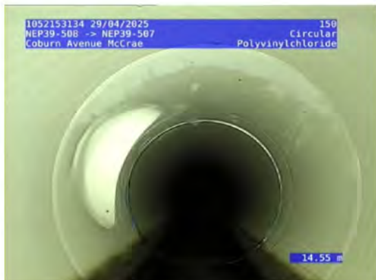
3, 00:03:50, 14.55 Junction, unlined, open, Height/Diameter (mm): 100 at 10 o'clock
