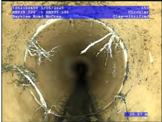
5, 00:06:46, 20.07 Cracking multiple or complex (s), at joint, width: 3mm from 12 o'clock to 12 o'clock
