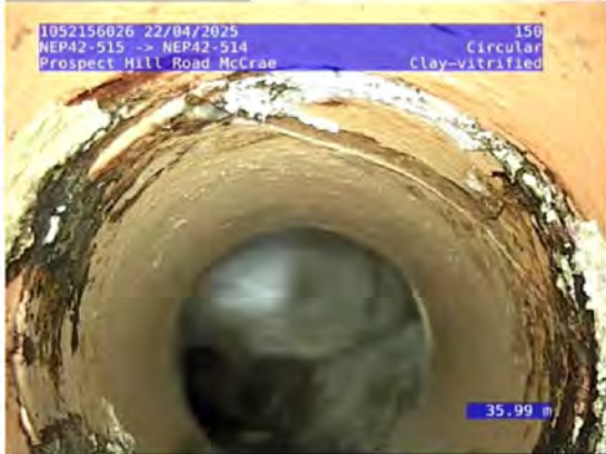
5, 00:11:00, 35.99 Infiltration, gushing, at joint from 11 o'clock to 1 o'clock
