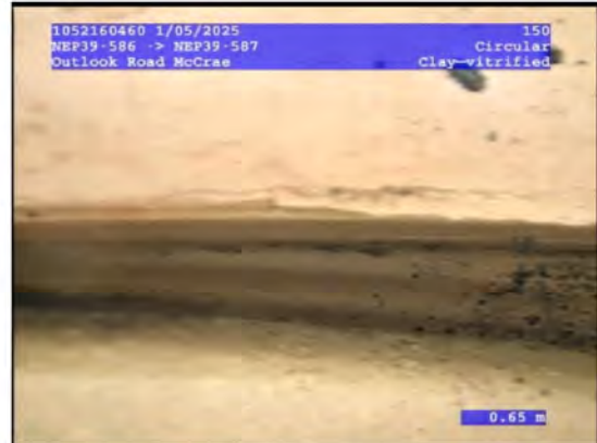
2, 00:00:40, 0.65 Joint displaced angular at 9 o'clock
