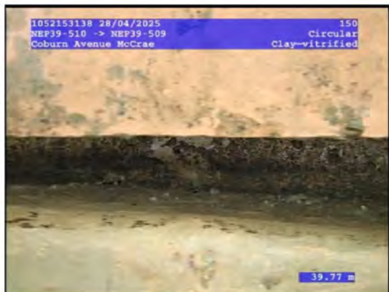
3, 00:13:07, 39.77 Joint displaced angular at 12 o'clock
