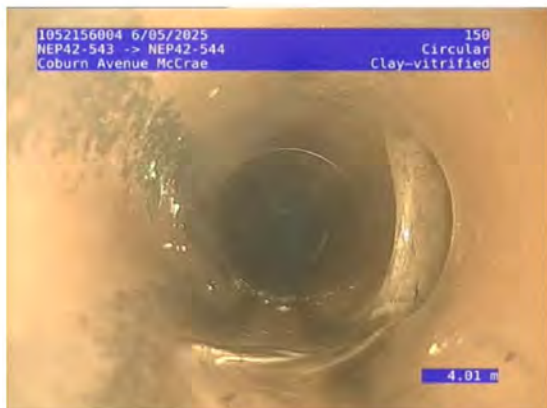
3, 00:04:03, 4.01 Junction, unlined, open, Height/Diameter (mm): 100 at 2 o'clock
