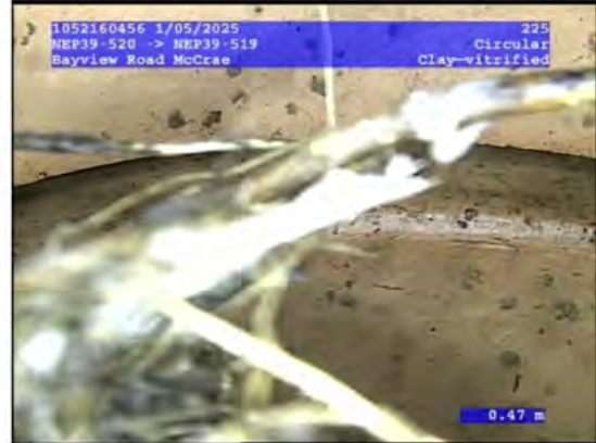
2, 00:01:26, 0.47 Recently cut interwoven mass of mostly fine roots leaving a beard of roots, Obstruction: 30%, at joint from 12 o'clock to 12 o'clock
