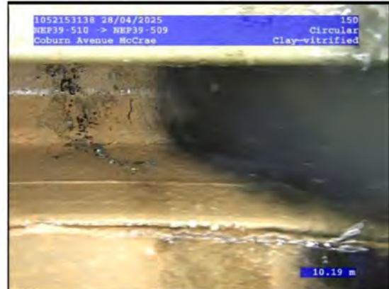
2, 00:04:32, 10.19 Joint displaced longitudinally, 10mm
