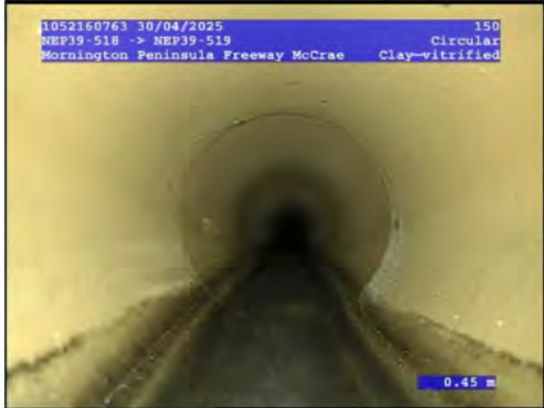
1, 00:00:40, 0.45 Water flow at constant depth, turbid or discoloured water, <5% / pulsating
