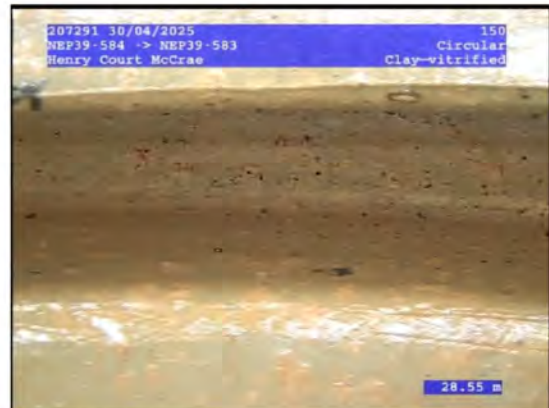
8, 00:13:38, 28.54 Joint displaced longitudinally, 20mm
