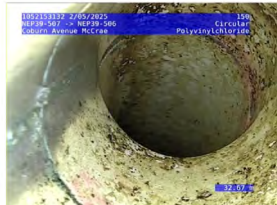
4, 00:08:17, 32.67 Junction, unlined, open, Height/Diameter (mm): 100 at 10 o'clock
