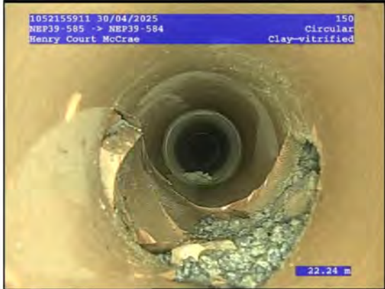
5, 00:10:21, 22.24 Conduit broken as a result of an exceptional event, e.g. external trauma, length of break: 500mm from 2 o'clock to 11 o'clock
