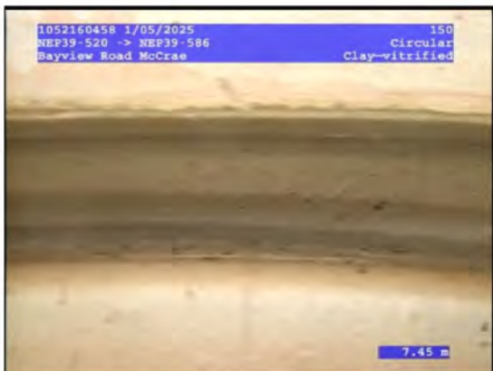
3, 00:03:02, 7.45 Joint displaced longitudinally, 10mm
