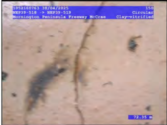
5, 00:32:33, 72.34 Longitudinal cracking, at joint, width: 1mm at 1 o'clock
