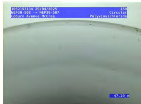
12, 00:13:18, 47.29 Joint displaced longitudinally, 40mm
