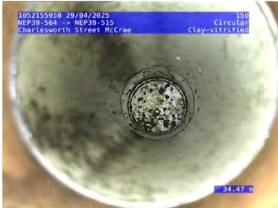
5, 00:12:16, 34.47 Junction, unlined, open, Height/Diameter (mm): 100 at 12 o'clock
