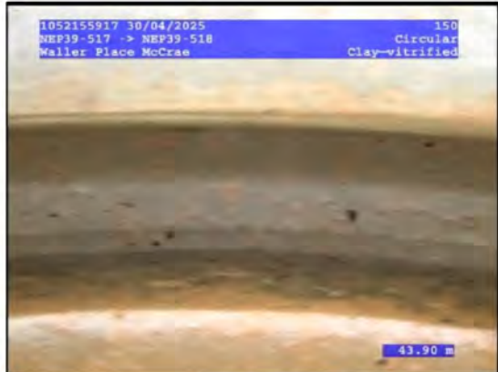
13, 00:17:28, 43.90 Joint displaced longitudinally, 20mm
