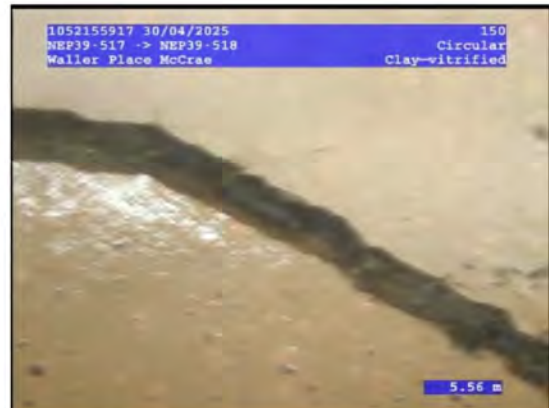
12, 00:05:03, 5.56 Circumferential cracking, width: 3mm from 12 o'clock to 12 o'clock / at connection
