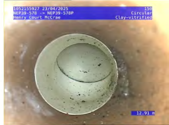
2, 00:04:59, 12.91 Junction, unlined, open, Height/Diameter (mm): 100 at 2 o'clock
