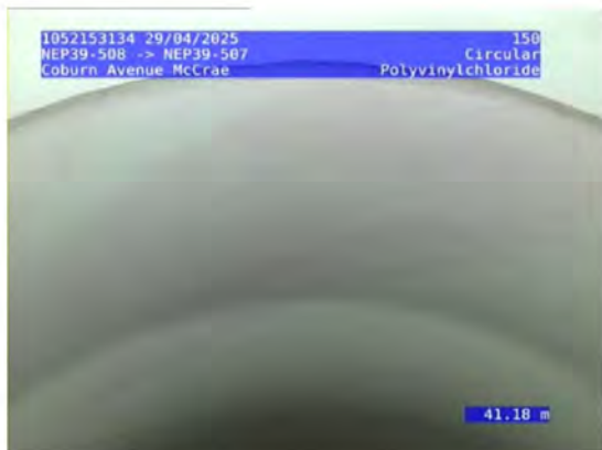
11, 00:12:08, 41.18 Joint displaced longitudinally, 50mm
