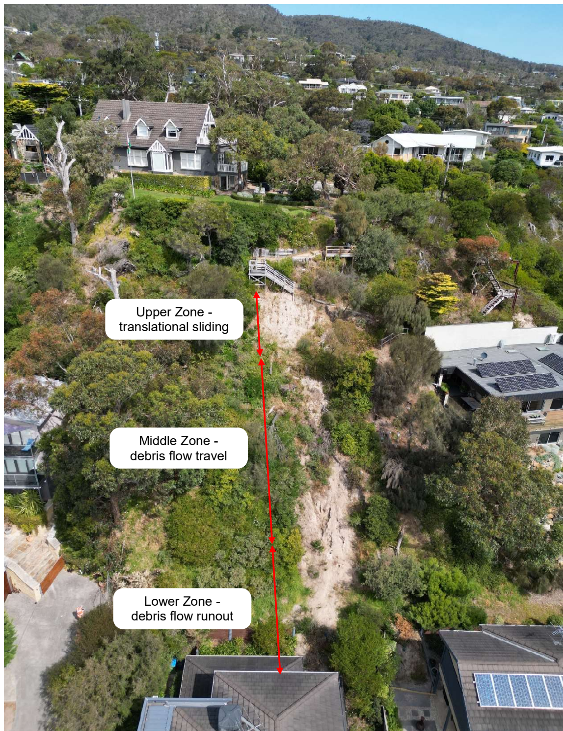
Photo 3 - Landslide Overview, with zones indicated
