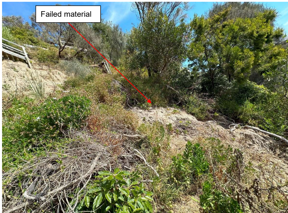
Photo 4 - Failed material still on slope
