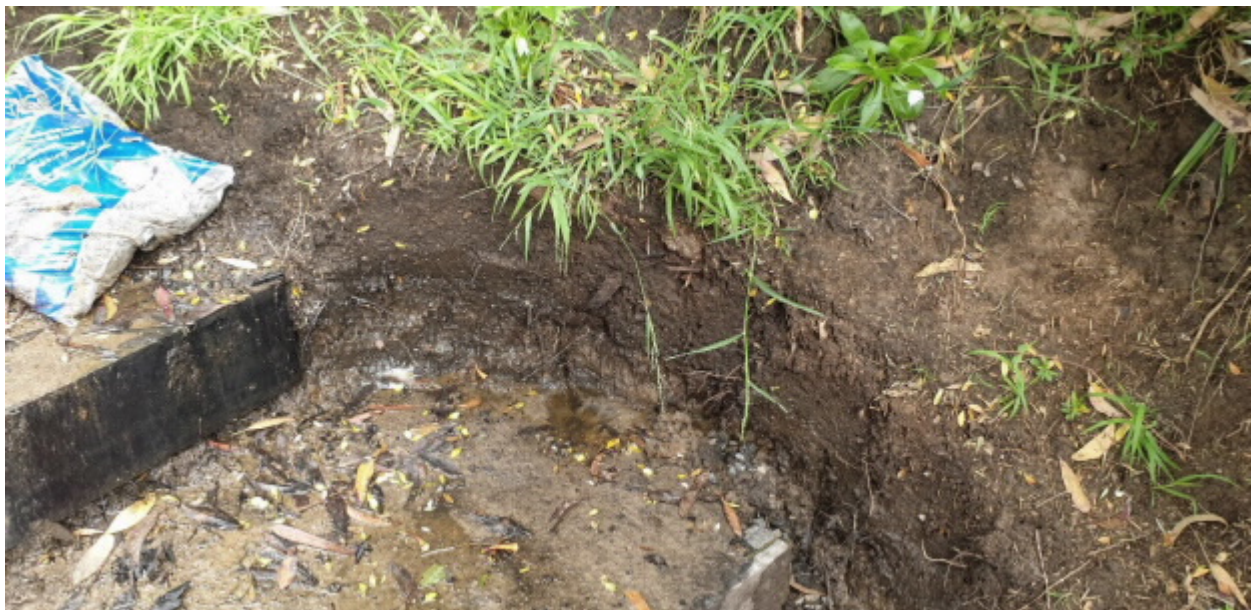
Figure 4-9: Water seepage on left side of site
