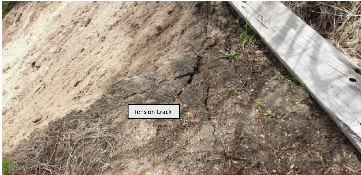
Figure 4-4: Tension crack on right flank
