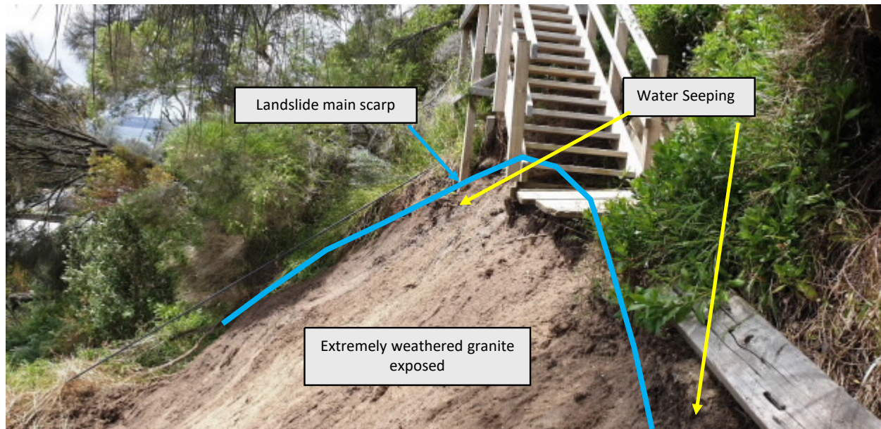
Figure 4-2: Main scarp of landslide
