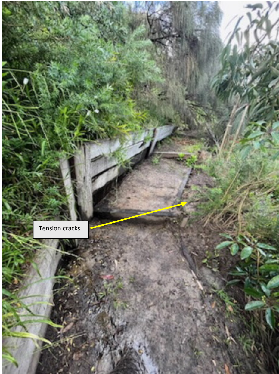
Figure 4-5: Leaning retaining wall and tension cracks on left flank
