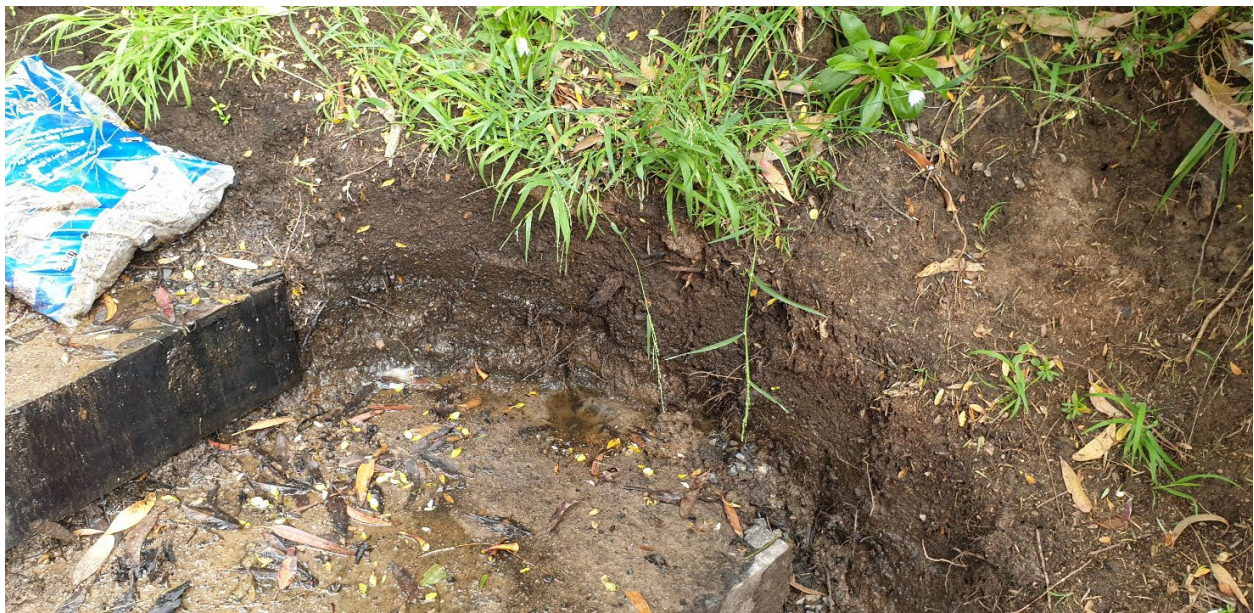
Figure 4-9: Water seepage on left side of site
