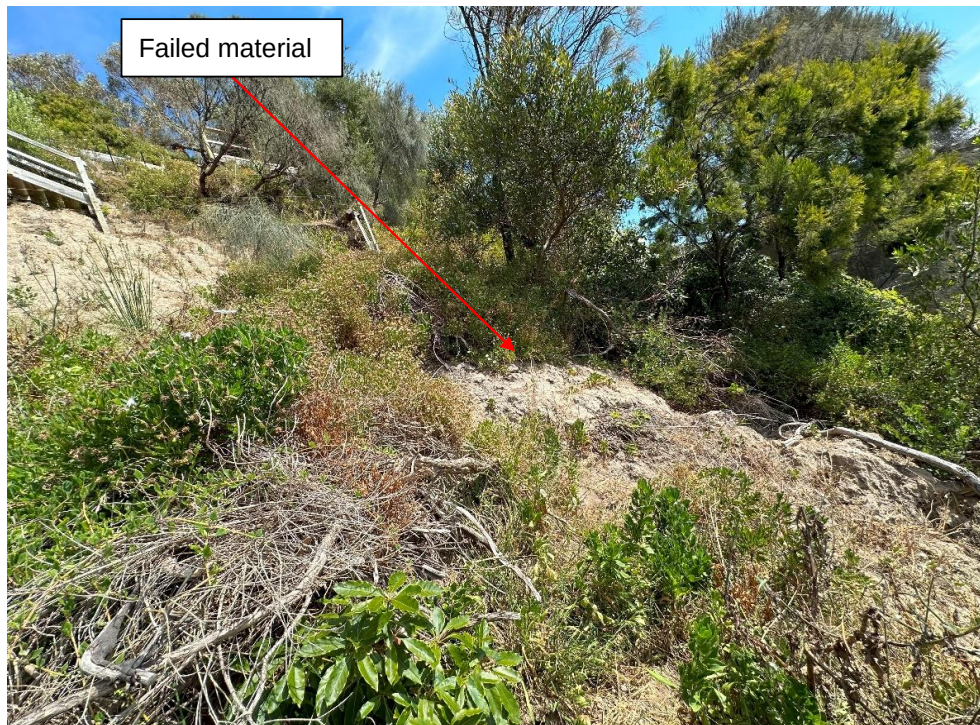
Photo 4 - Failed material still on slope
