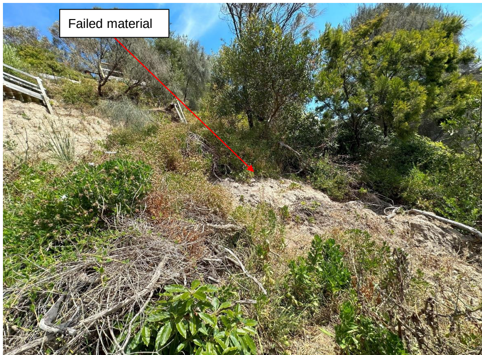
Photo 4 - Failed material still on slope
