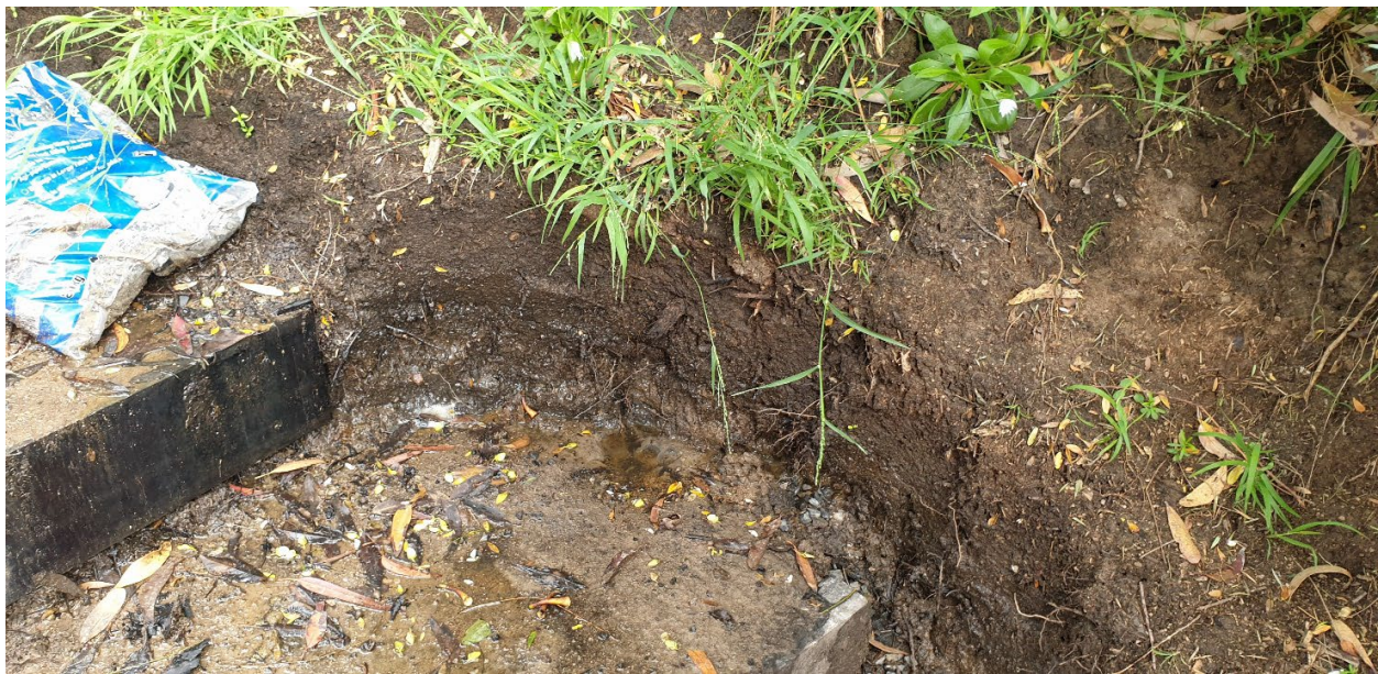
Figure 4-9: Water seepage on left side of site
