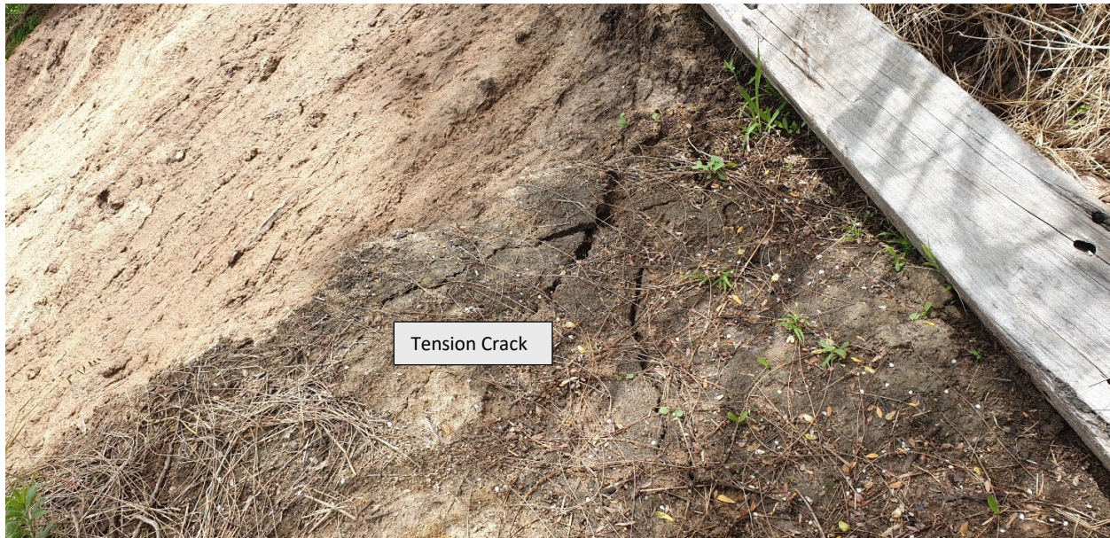
Figure 4-4: Tension crack on right flank
