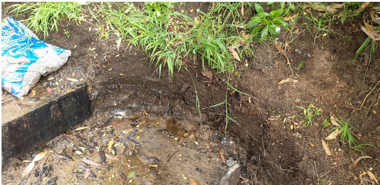
Figure 4-9: Water seepage on left side of site
